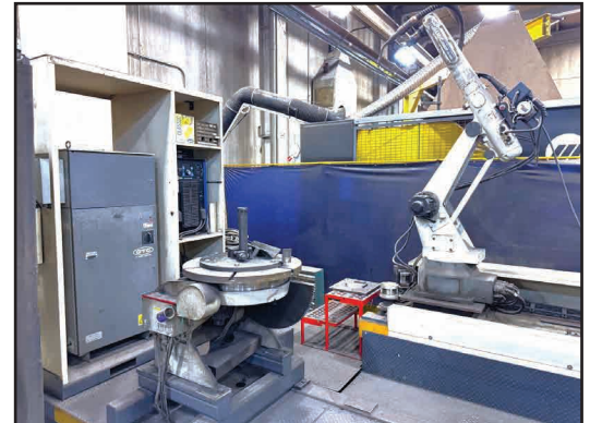
OTC DAIHEN ROBOTIC WELDING CELL
